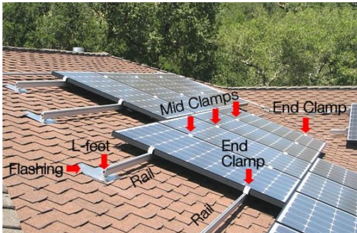
Figure 4-1: Mounting arrangement of PV panels
